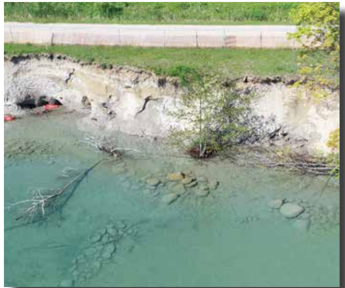
Erosion damage at Bluff Road
